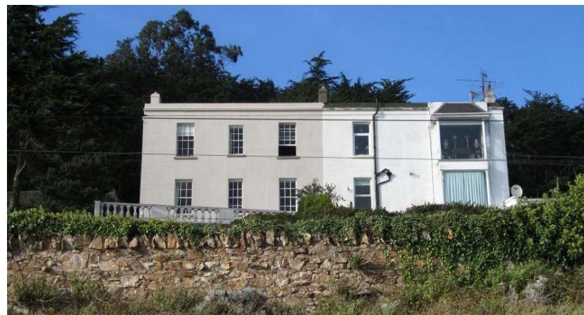
Unsympathetic alteration of window formats and addition of surface mounted pipes.
