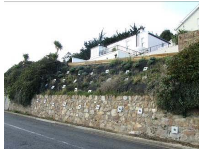
Unsympathetic engineering works to retaining walls
