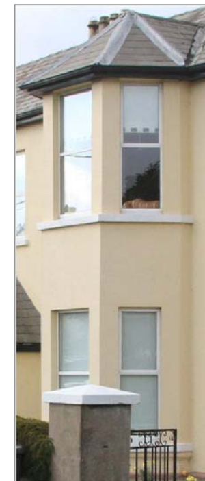
Plate 7: Bay window on St. Michael's and double bay to front of Gordon Ville
