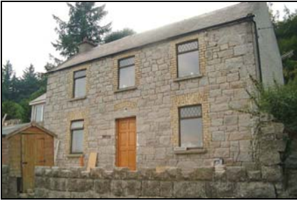
Double Storey Victorian House with stripped render and replacement windows, Barnacullia Historic Settlement Node
