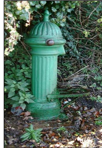
Low Level Water Pump, Ballyedmonduff / Barnacullia Road Axis
