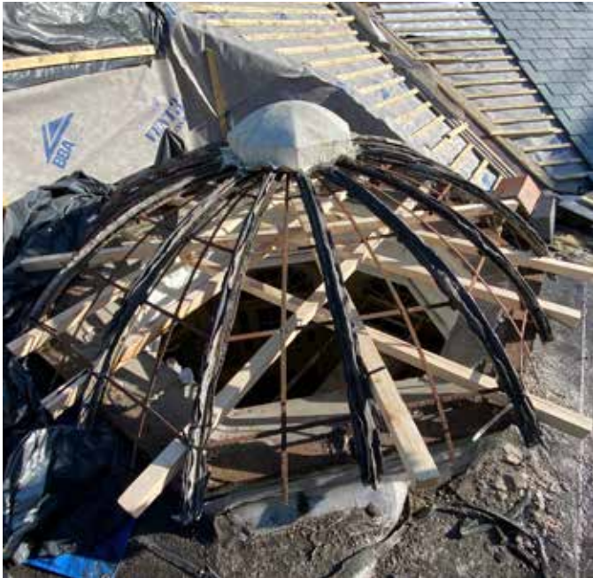
DL Carnegie Library Rooflight Repair (Before)
