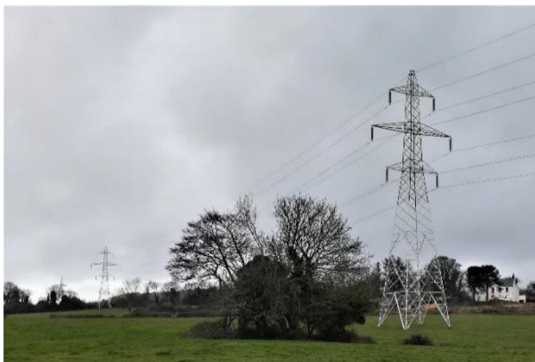
Plate 12.8 - the Arklow-Carrickmines ESB Pylons
