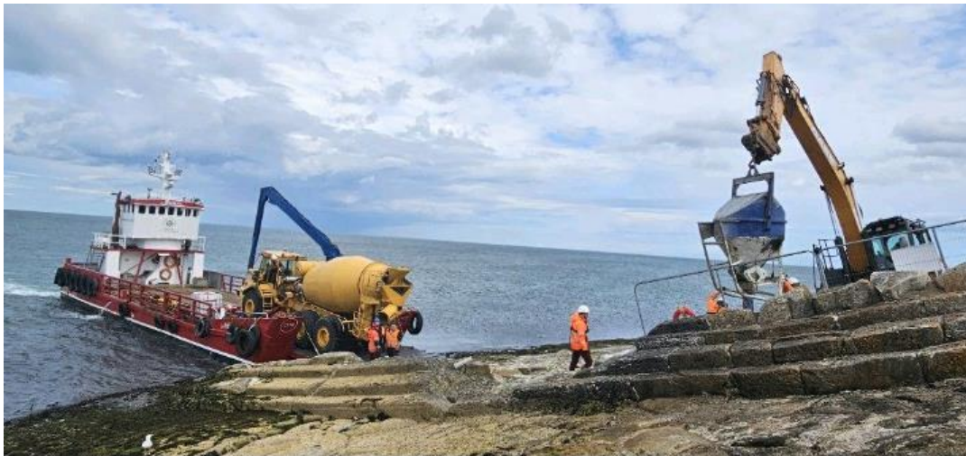
A “landing craft” delivering concrete to the back of the East Pier.
