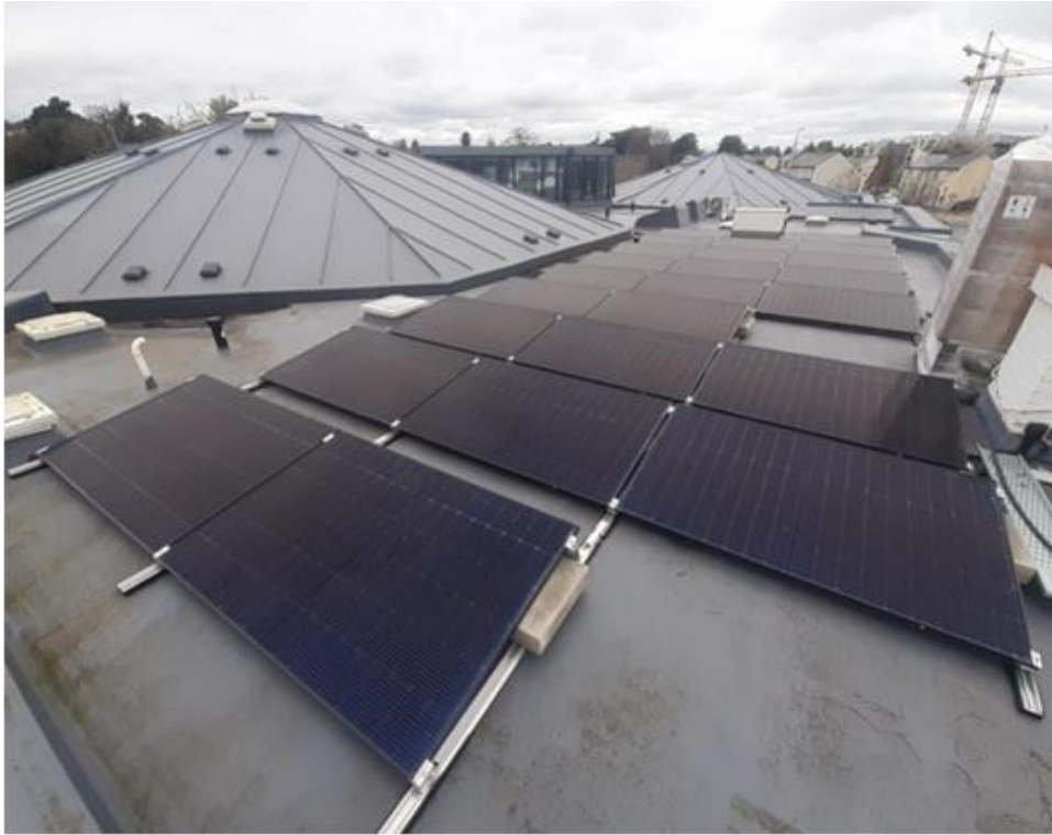
Deansgrange Library roof with Solar Panels installed
