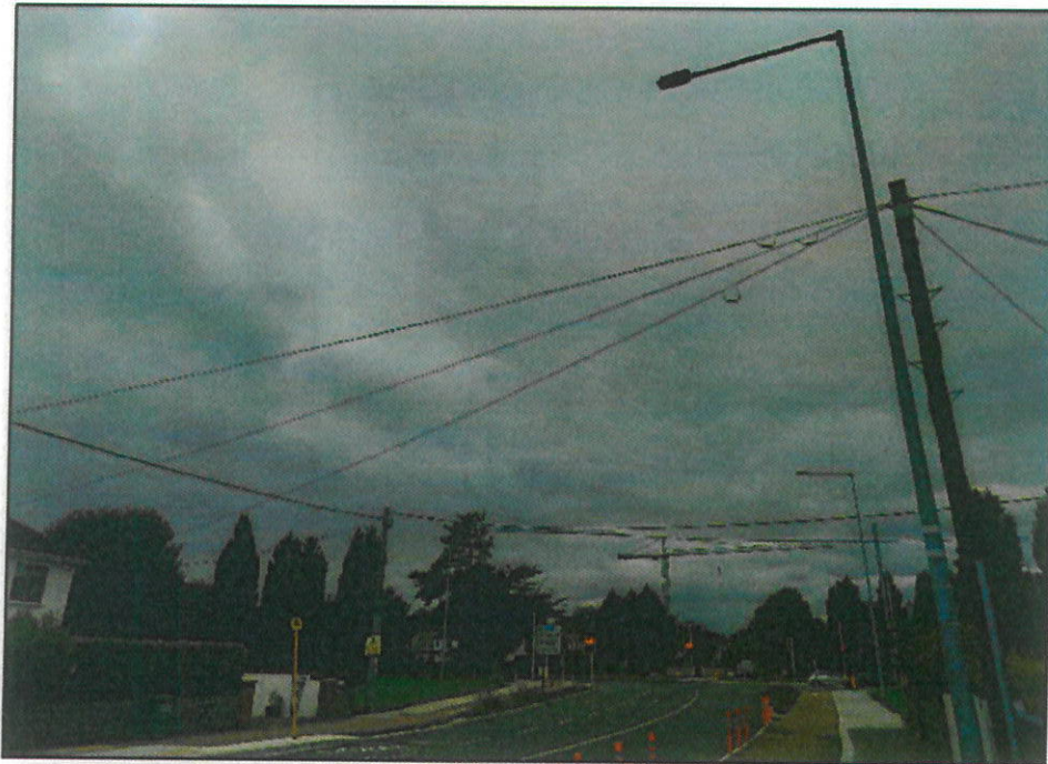
VRP10 - WITHOUT SOLUTION IN PLACE
