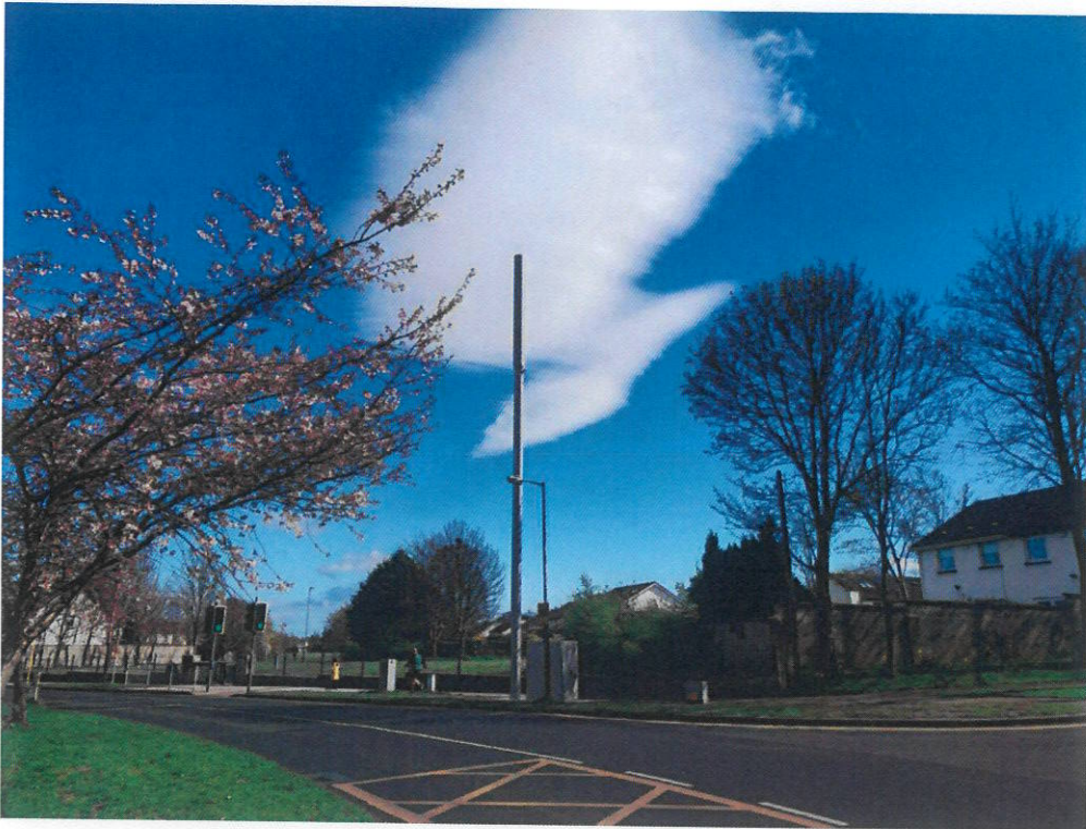
15m Streetworks Solution at Knocklyon Road Installed under S254 Licence from SDCC
