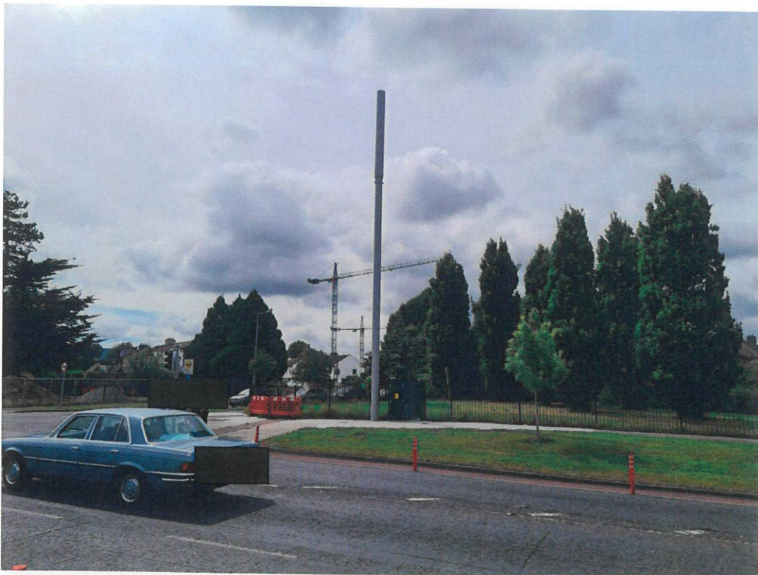
15m Street works at Drummartin Road Dublin 14, installed under S254 licence from DLR Co Co
