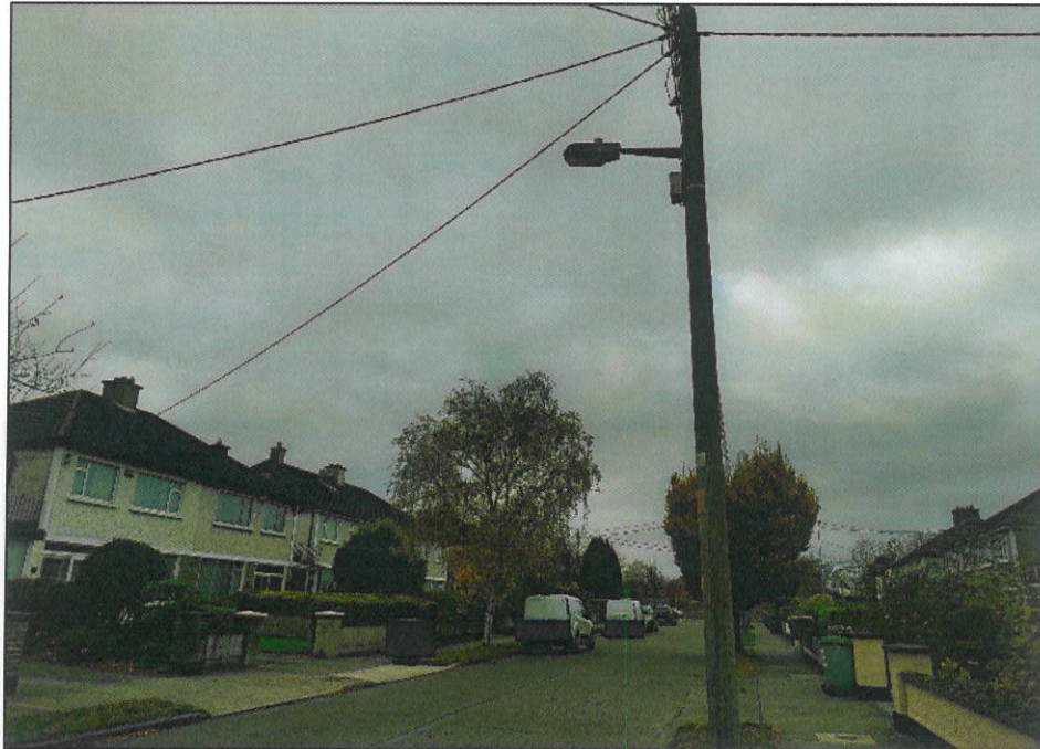
VRP4 - WITHOUT SOLUTION IN PLACE
