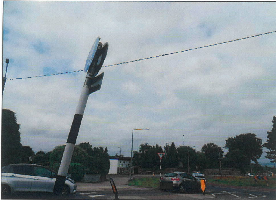
VRP3 - WITHOUT SOLUTION IN PLACE
