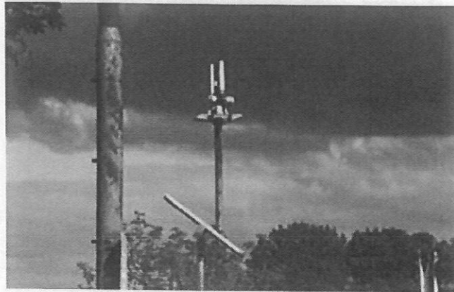
Image 4 Existing eir Mobile pole in Nutgrove ComReg Site ID: 1210
