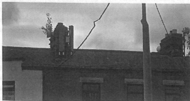
Image 5; existing eir installation ComReg Site ID: 3311
