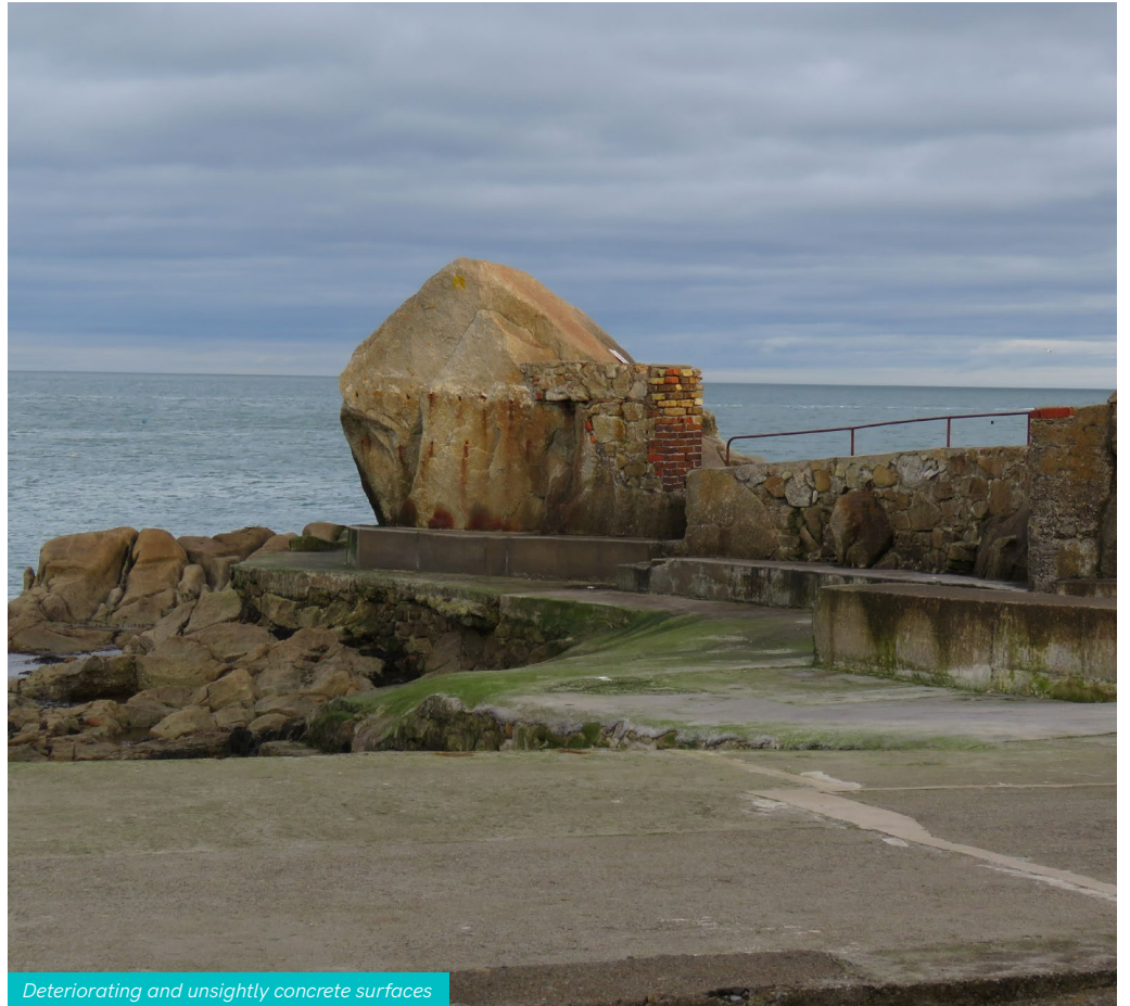
Deteriorating and unsightly concrete surfaces
