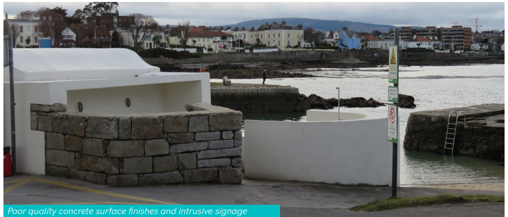
Poor quality concrete surface finishes and intrusive signage
