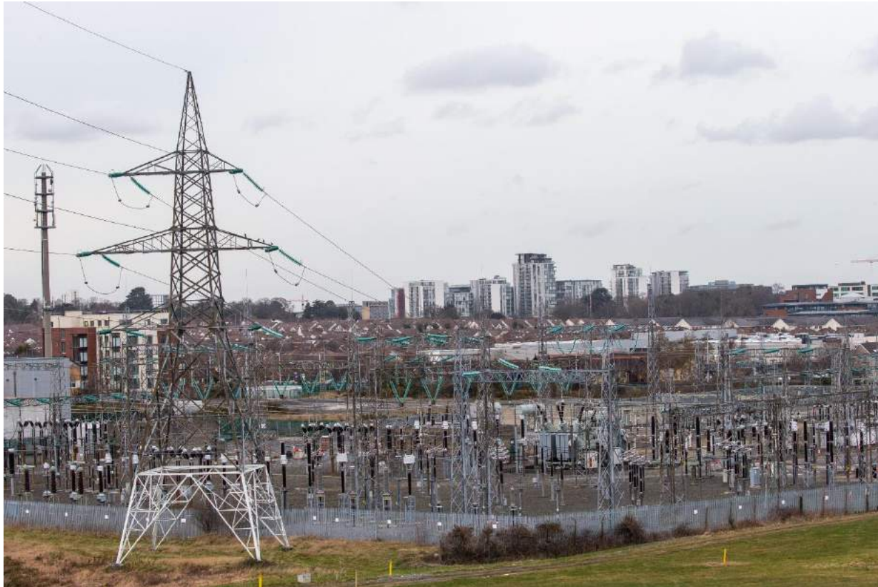
Figure 10.2 – 220kV substation at Ballyogan South, viewed from former landfill
