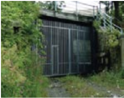
Tunnel entrance near Royal St. George Yacht Club. This area requires maintenance having suffered neglect over the years.
