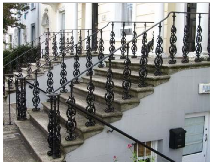
Stucco façade (top) and ironwork and steps (above). View of No.s 16-17 Adelaide St., left
