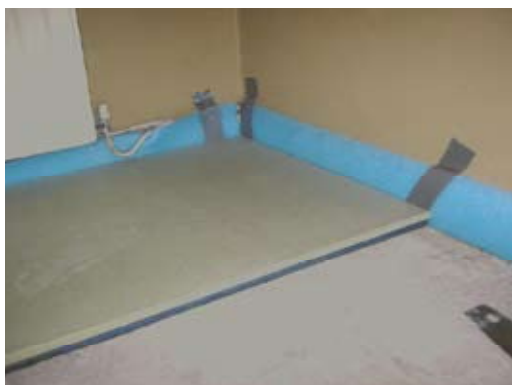
Fig 5. Addition of floor insulation to a modern concrete floor. Lister Housing Co-operative.
