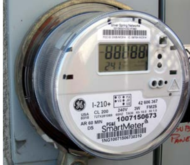
Figure 245. Smart meter. Source: www.deepresource.wordpress.com .
