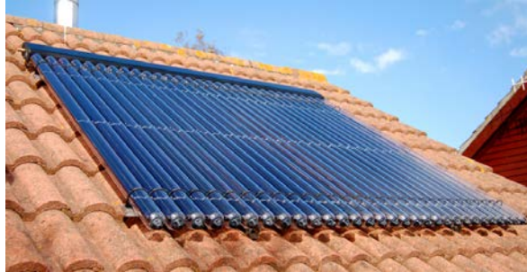
Figure 239. Solar thermal evacuated tubes in a building. Source: www.yougen.co.uk .
