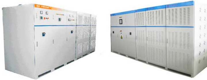
Figure 249. Energy storage station. Source: www.ecopowernt.com.au .
