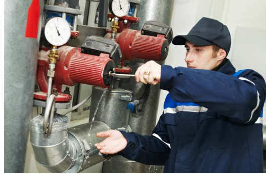
Figure 44. Maintenance and inspection of water pumps. Source:www.electrobombasmanogil.com.
