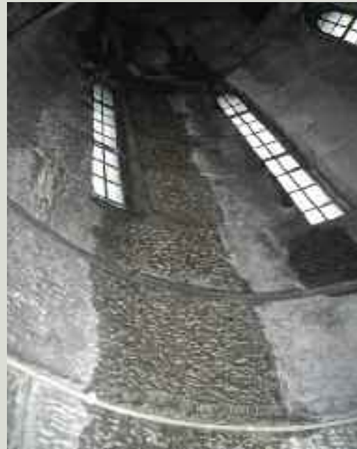
Difficulty of access no doubt contributed to lack of maintenance of this church tower, resulting in ingress of water to saturation level in the masonry. This will lead inevitably to serious damage unless it is remedied
