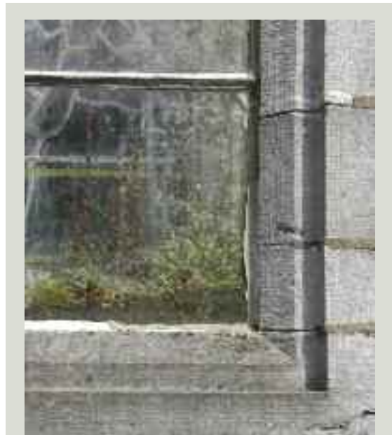
Sealed, or inadequately ventilated, storm glazing provides an opportunity for the growth of vegetation, which damages the stained glass as well as being unsightly
