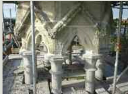
This Bath stone turret, which is also a bell-tower, is in a highly exposed location. Several stones cracked due to rusted cramps and the poor condition was exacerbated by previous misguided cementitious repair. New stainless steel collars and ties were fitted and the turret was repointed
