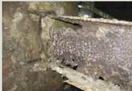
The extent to which driving rain and lack of a protective coating can damage bell supports is shown by this badly corroded steel beam
