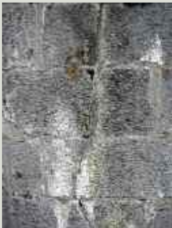
This wall has become overly rigid due to the use of cement mortars, which resulted in the mortar becoming harder than the stone. Structural movement in the church is seen in the vertical cracking through the ashlar stones rather than the mortar
