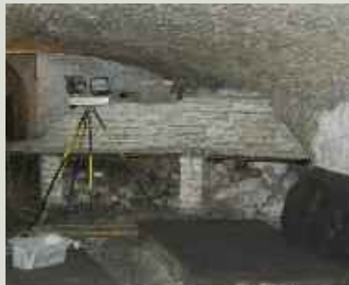
Inspecting a crypt presents risks such as trip hazards, toxic fumes, asbestos and rodent or fungal infestation. Personal protective equipment and adequate lighting are essential to reduce the risk of accident to the inspector or damage to the structure
