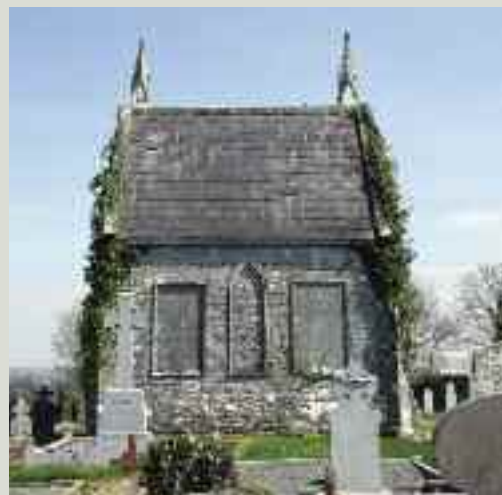
Some mausolea are shaped like miniature churches, containing high quality architectural details and materials. Mausolea require sufficient maintenance to prevent them slipping into a state of neglect, damaging the remains within and endangering visitors to the graveyard
