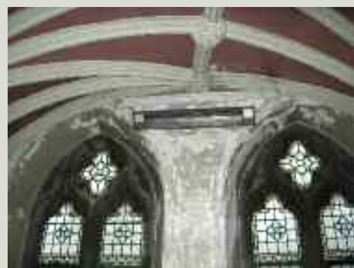
Church lighting and heating systems may evolve on an ad-hoc basis as funds become available. In this case, strip lights and electric bar heaters were fitted to some of the aisles. Conservation works to the church will include the removal of these fittings and repairs to the roof above to eradicate the damp in the wall
