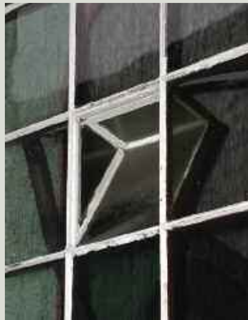
Original ventilators in the glazing should be repaired where necessary and opened after church services. Care should be taken in operating the mechanism to avoid damaging historic glass
