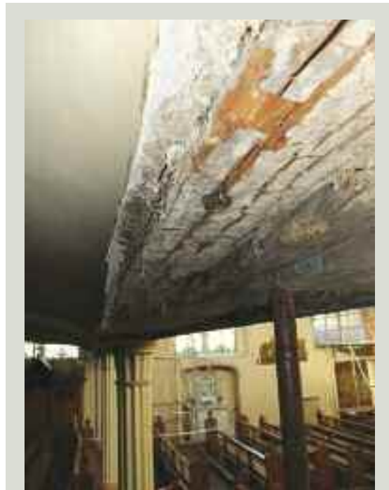
Regular inspections and scheduled maintenance work should prevent rot from taking hold to the degree that it causes structural damage, as has happened to this beam which supports an organ gallery
