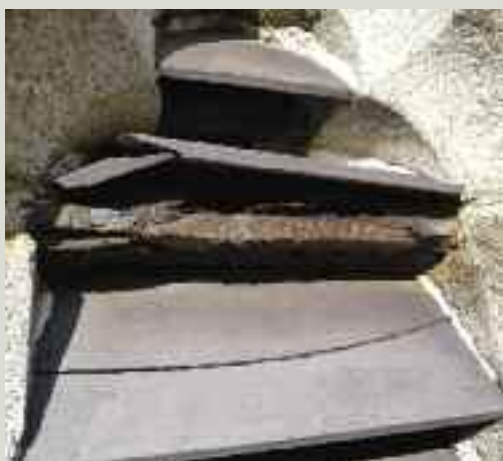
Embedded metal tie bars in this bell tower corroded and expanded, causing fractures in adjacent granite and slate louvres. Part of the repair solution involved installing a cathodic protection system to reduce the corrosion rate of the embedded ironwork
