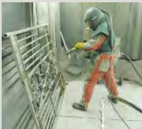
Blast cleaning ironwork in a blast chamber (Image courtesy of Historic Scotland)
