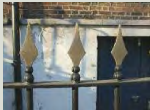
The original cast iron finial is depicted on top. Mild steel replacement finials are shown below. These are flat and poorly designed in comparison to the original and have been individually welded onto the rail
