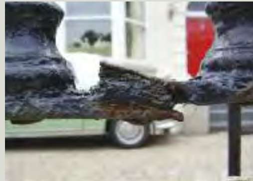
Corrosion developing at a scarf joint
