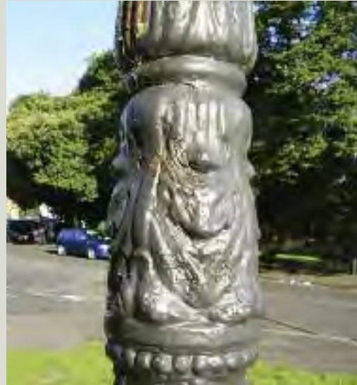
Over-thick application of paint will obscure detail and result in less effective protection
