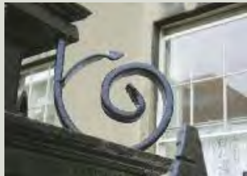
It is important to choose an experienced craftsman to avoid inappropriate repairs. The replacement scroll in the lower image has been crudely formed and bears little resemblance to the finely-crafted original feature on a neighbouring property in the top image
