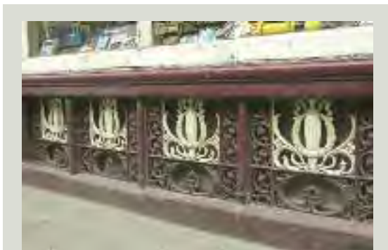
Routine maintenance to ironwork, such as this attractive cast iron stall riser to a shopfront should include gentle washing using a minimum amount of water to remove accumulated dirt
