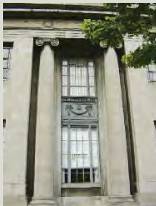
The National Concert Hall, Earlsfort Terrace, Dublin. Cast iron windows and spandrel panels became increasingly widespread from the start of the twentieth century. This example was supplied by the Scottish firm Walter Macfarlane & Co. Ltd in 1914
