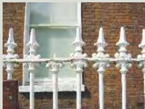
Missing cast iron finials, collars, and husks are common due to the development of galvanic corrosion between these decorative elements and the wrought iron bar that they are usually placed over. It is generally possible to cast and fit new finials, although husks and collars below the top rail can be more problematic to replace due to the need to dismantle the railings in order to place them in position
