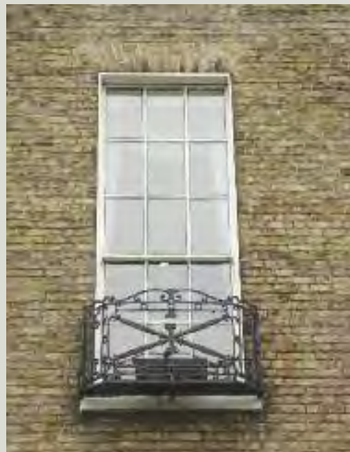
Due to their position and the potential for injuring people below, balconies and balconettes should be periodically inspected to ensure that they are secure
