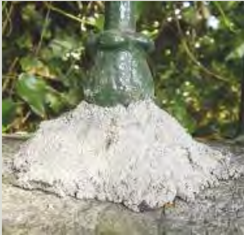
Concrete is not an appropriate material for the repair of ironwork, particularly in combination with stone
