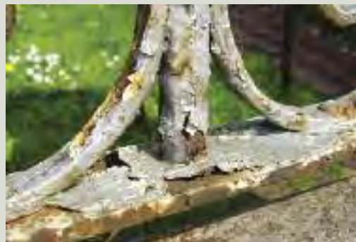
Broken, flaking paint traps and holds water to the iron, preventing it from drying out properly, and can lead to corrosion. Areas of chipped paint are not as significant a threat so long as the iron is in an exposed location and is able to dry out. Nevertheless, such chips should be treated as soon as possible to prevent rust from forming
